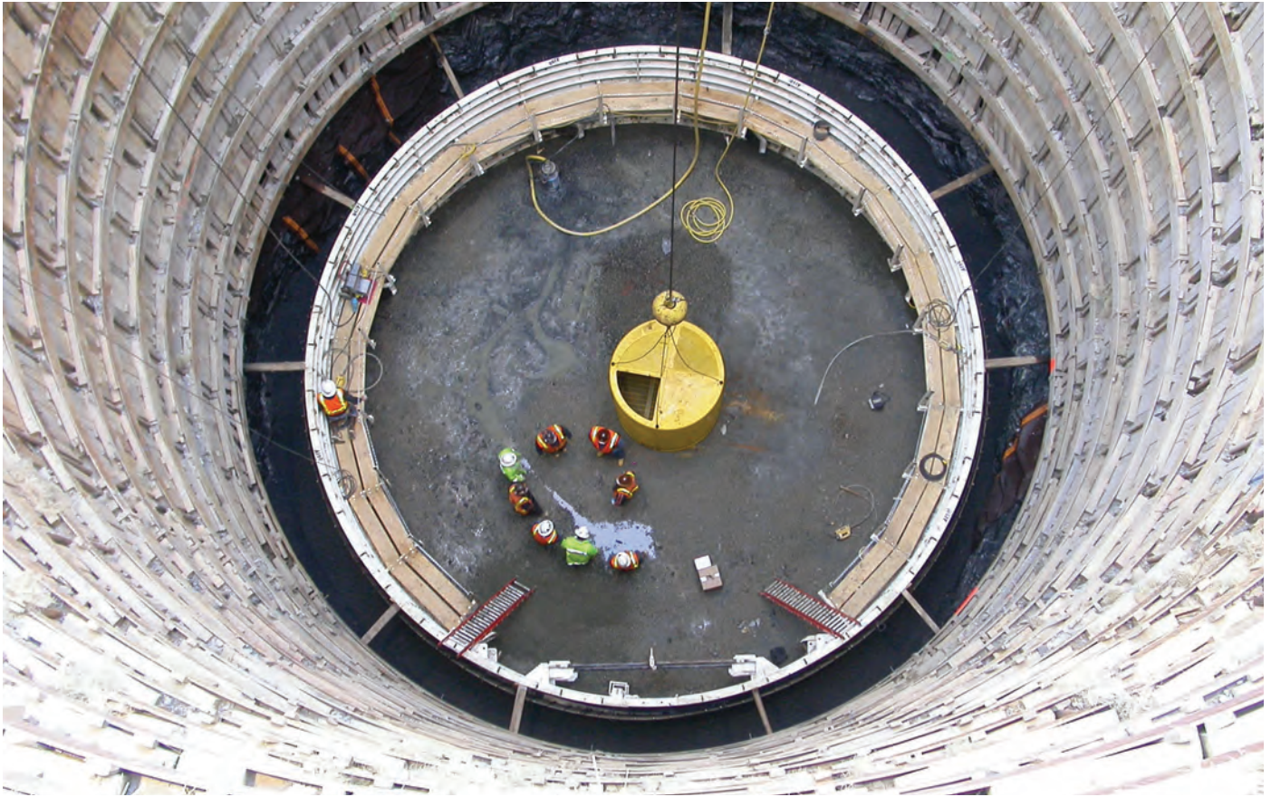
West Area CSO Storage Tunnels and Pumping Station, Atlanta, Georgia: Primary responsibility for design of the tunnel and shaft linings, including preparation of tunnel and shaft specifications.*
