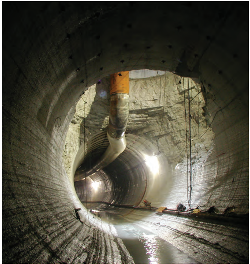
Elm Road GS Water Intake Tunnel, Oak Creek, Wisconsin: Hatch was responsible for all engineering, procurement, and construction necessary to provide the Intake Water Tunnel.
