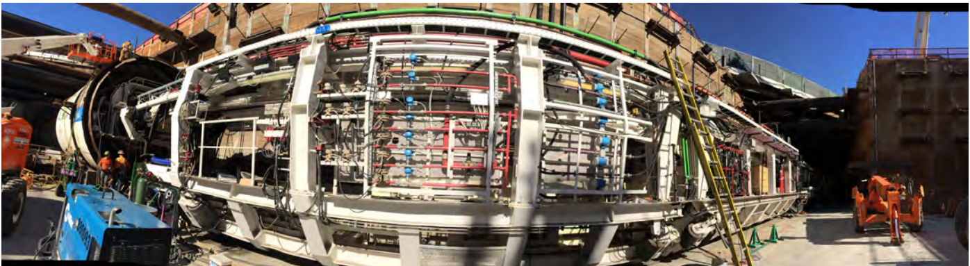
Regional Connector Transit Corridor, Los Angeles, California: TBM assembly prior to launch. *
