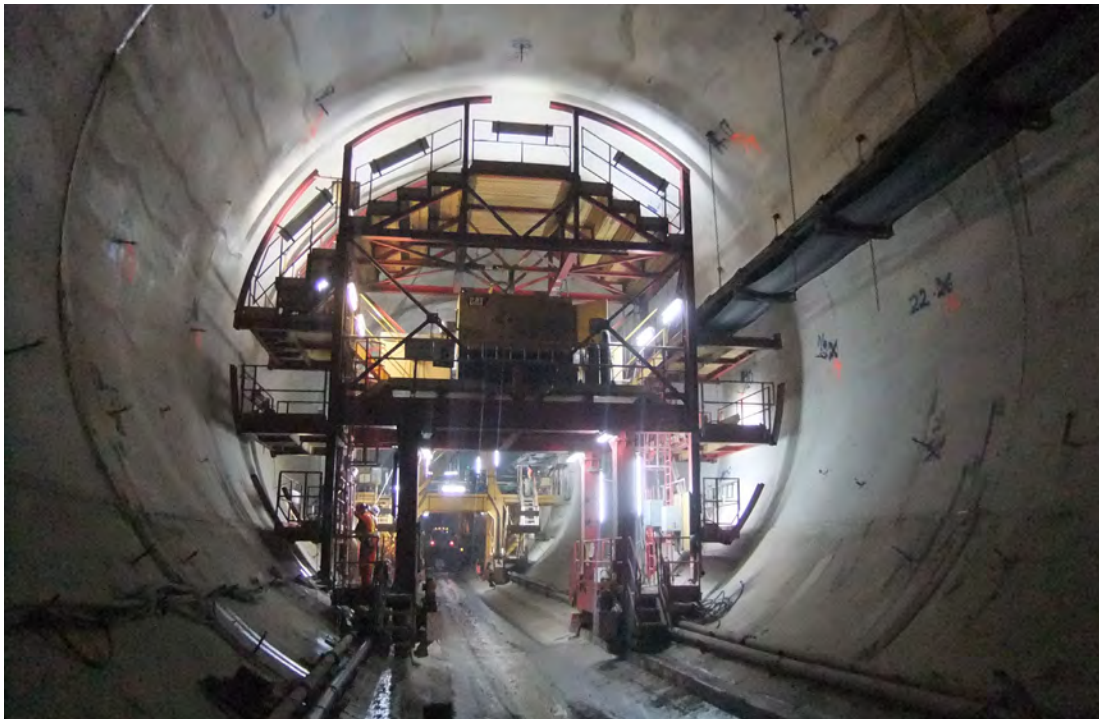
Niagara Power Tunnel, Niagara Falls, Ontario: As Owner's Representative Hatch developed the concept design and set out the owner's mandatory requirements. (Photo provided courtesy of Ontario Power Generation Inc.)
