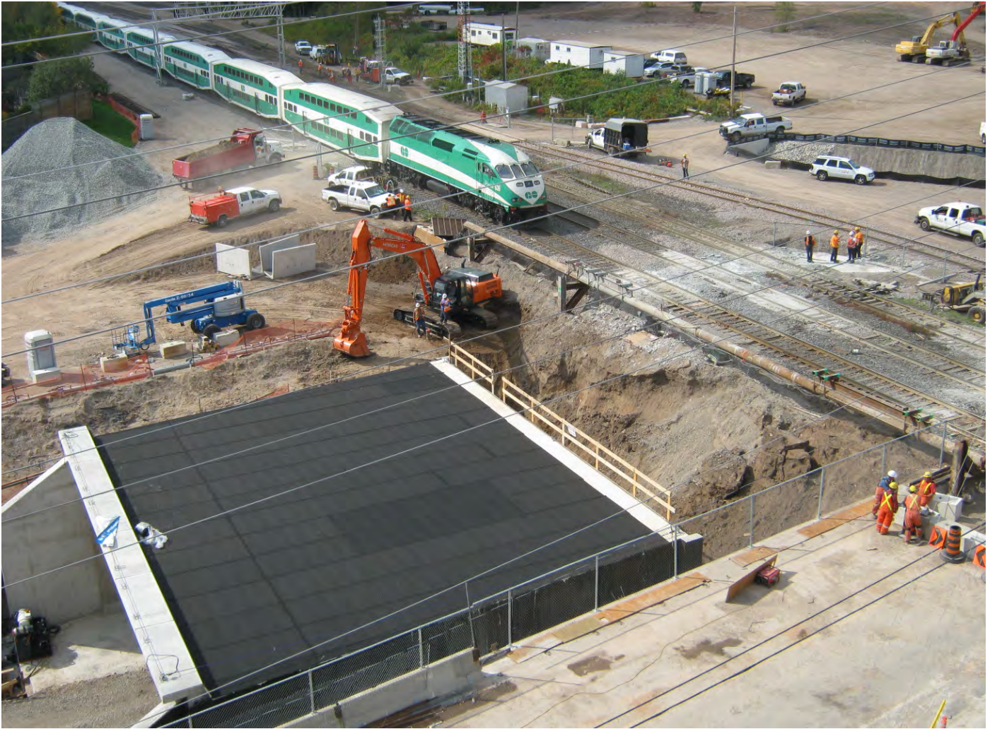
King Road/CN Grade Separation, Burlington, Ontario: Prime consultant responsible for the entire project.
