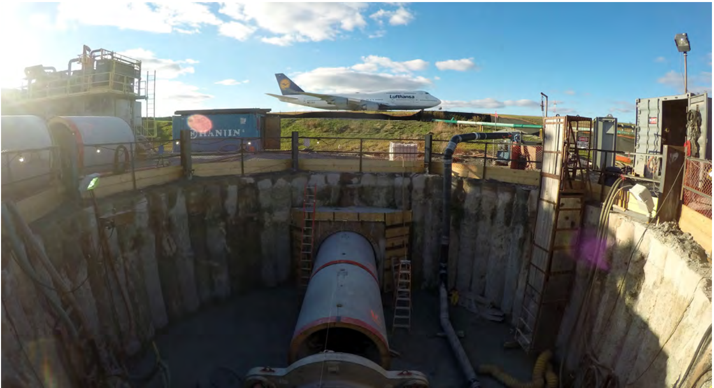
Etobicoke Creek Trunk Sanitary Sewer Twinning, Toronto, Ontario: Etobicoke Creek Trunk : Primary consultant providing preliminary and detailed design of the trunk sewer
