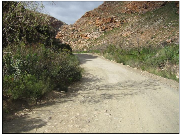
Figure 5: Current river crossing at km 47.2. Note eroded road surface in foreground.
