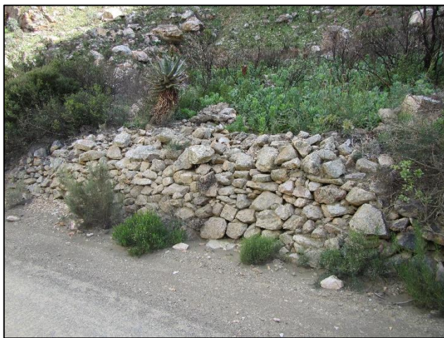
Figure 34: View of the stone retaining wall located along the road at waypoints 674-675.
